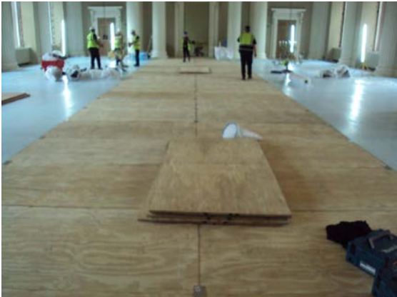
Figure 6: Substantial floor protections are put in place ready for the giant scaffold
