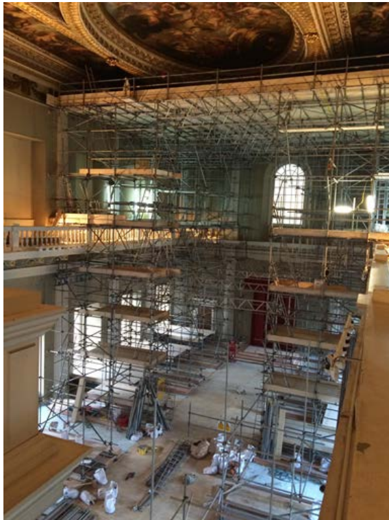
Fig. 8: The scaffold will accommodate work to the windows and ceiling is built in three phases
