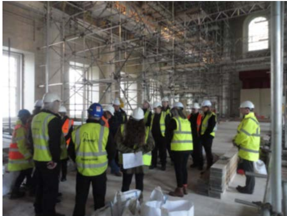
Fig. 11: Conservators and Surveyors briefing the asbestos removal team who will work in close proximity above and below the paintings and coffering
