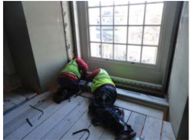
Fig. 9 Final preparation of the new window frames ready to receive the new window
