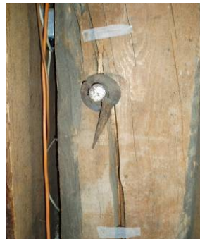
Historic bolting through front and rear columns. Splits/shakes in structural columns
