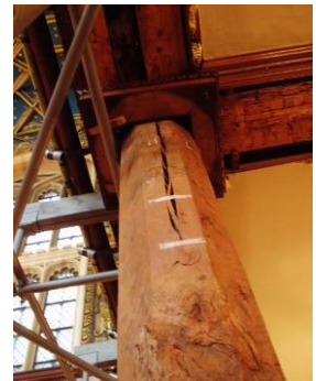
Splits and shakes to top of column.
